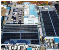
Solar Power Generation Facilities at the Cheonan Campus
